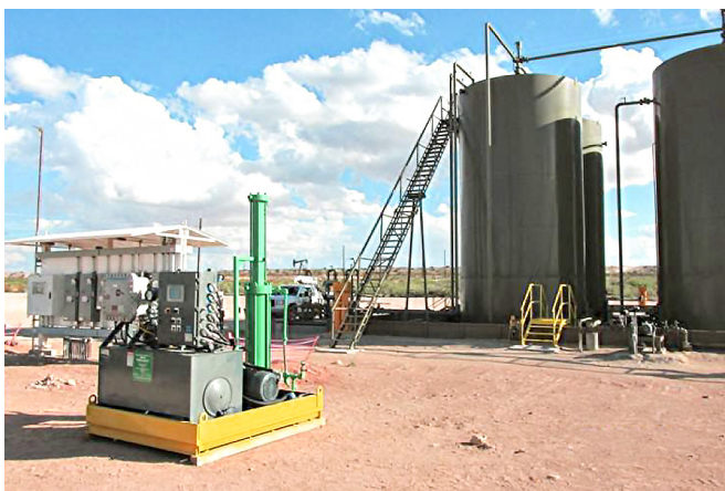
Fig. 4. Typically, the HyBGC VRU unit operates at service dependability rates in excess of 99.4% per year.
