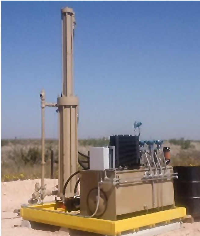
Fig. 1. The HyBGC does not increase the discharge temperature of the gas as severely as its counterparts, allowing gas to be discharged directly to sales lines.
